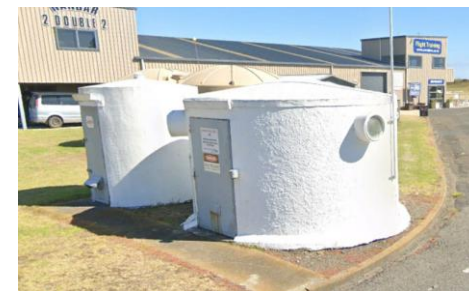
Figure 7-7: Aerodrome lighting control housing
